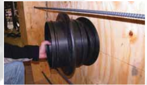
3. Cut the Infinity® wall sleeve \frac{3}{4} " shorter than the wall thickness (+/-1/4"), then insert the sleeve over the locator cap.
